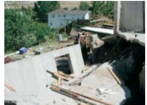
Basement and foundation straddling the main scarp. The wood frame portion of the house was moved off the foundation on August 25, 2001.
