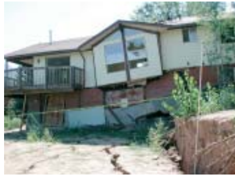
House straddling the main scarp. The house was demolished on August 27, 2001.
