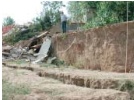
Main scarp height of 9 feet with the remains of demolished house at left. Note the displacement increase from photo above.
