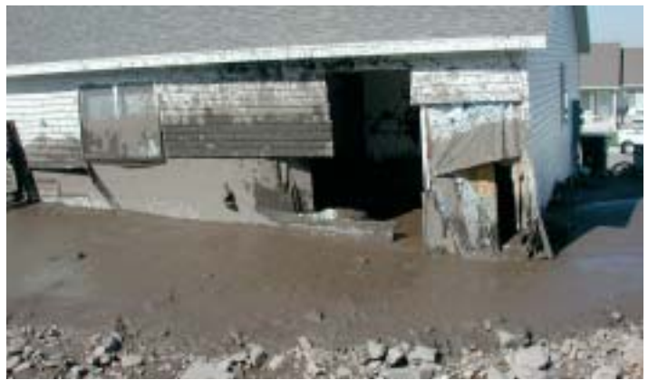
The debris flow broke through the back wall of this house on Peach Street in Santaquin.
