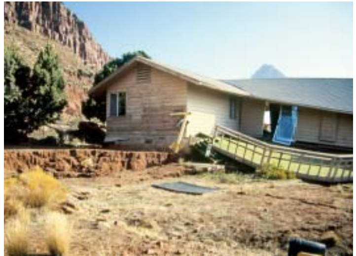
A landslide caused by the 1992 St. George earthquake destroyed this house in Springdale.
