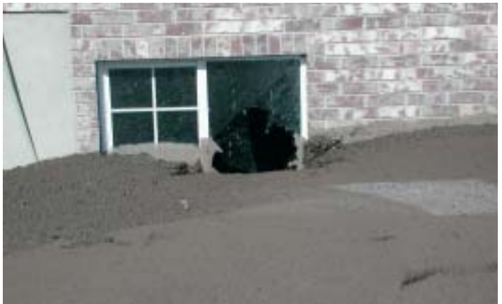
The debris-flow impact broke through the basement window of this house on Apple View Street in Santaquin.
