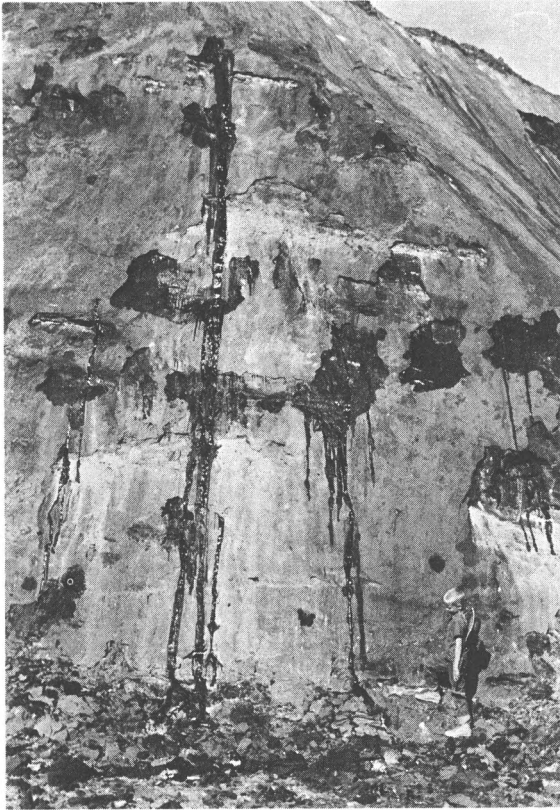
Figure 4. View of a tar seep in the County Asphalt Pit on Asphalt Ridge. The hot sun on the rich bituminous beds causes the liquid bitumen to "sweat" & run down the face of the quarry. Note that the bituminous beds quickly weather to a light gray color masking the rich black color beneath. The boy in the picture is the author's son, Bobby.
