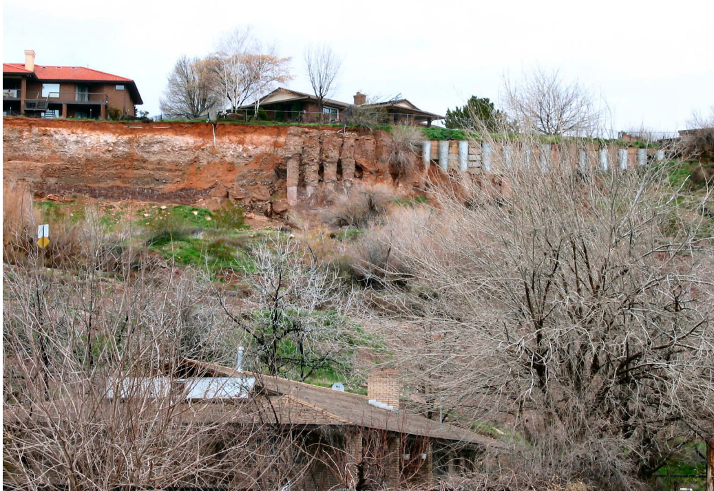
Figure 22. First recognized in the early 1980s, the Truman Drive landslide developed in the Petrified Forest Member of the Chinle Formation, and has remained intermittently active to the present; major periods of reactivation occurred in 1992 and again in 2002–03 (Lund and others, 2007b). In an effort to stabilize the main landslide scarp and prevent further damage to homes and utilities, large-diameter boreholes were drilled along the top of the slide, culverts reinforced with rebar were inserted in the boreholes, and the culverts were filled with concrete to create “soldier piles.” However, the landslide has continued to enlarge, destroying several of the piles. Large landslides in Petrified Forest strata are common, especially where exposed in steep hillsides protected from erosion by resistant cap rock or terrace gravels. The brightly colored swelling claystone of the member also exhibits a high shrink-swell potential (it expands when wet and shrinks upon drying), commonly leading to road and foundation problems.
