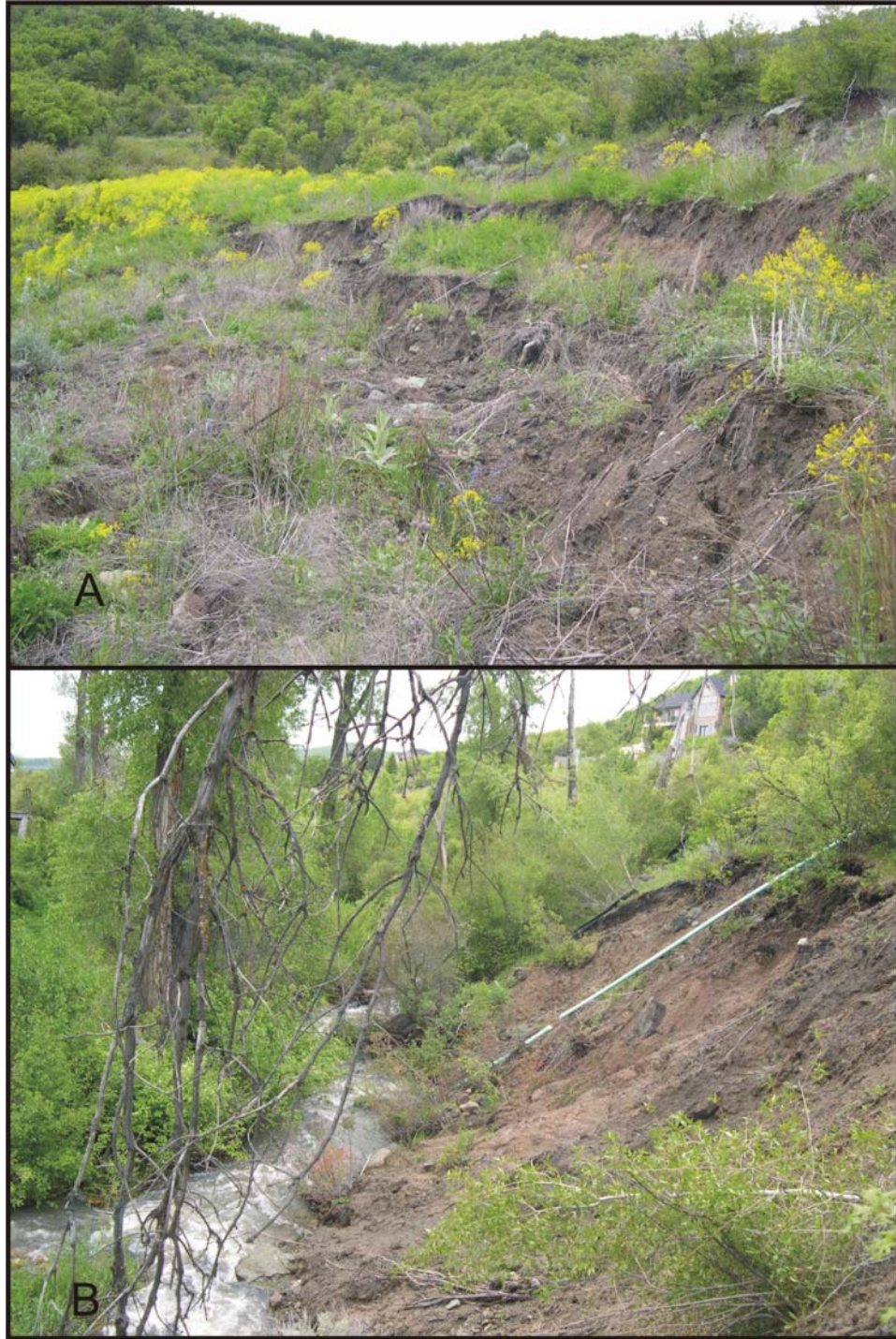
Figure 4. Northern Sewer-Line landslide. (A) View to the south-southwest of main scarp zone of the landslide. Top of main scarp was only a few feet from the east edge of the sewer-line corridor. (B) View to the south of toe of the landslide along Gordon Creek. Note drainpipe exposed along south flank of landslide.
