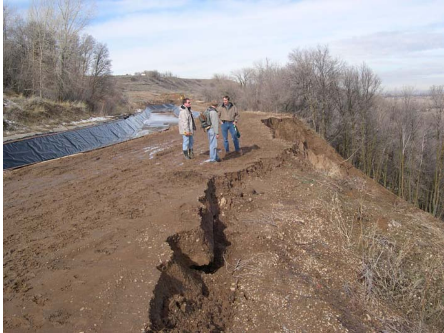
Figure 5. View west of the landslide crown, the Davis-Weber Canal, and the landslide main scarp. Eastward extension of the main scarp in the foreground indicates movement in the slope east of the landslide.
