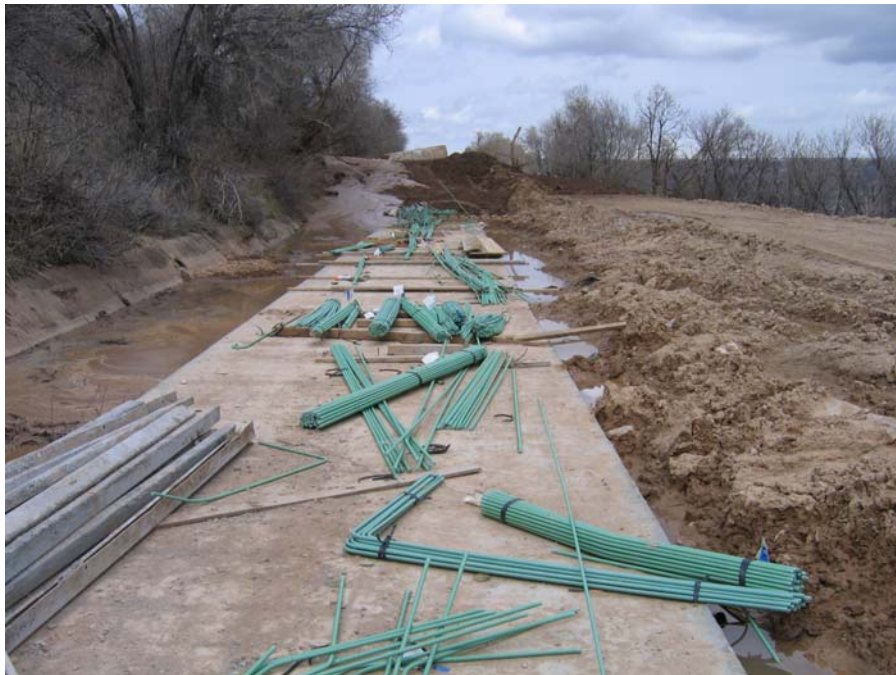
Figure 9. View looking northwest of Davis-Weber Canal showing landslide material deposited on the box culvert and canal access road. Following the landslide water and sediment flowed into the canal left of the box culvert.
