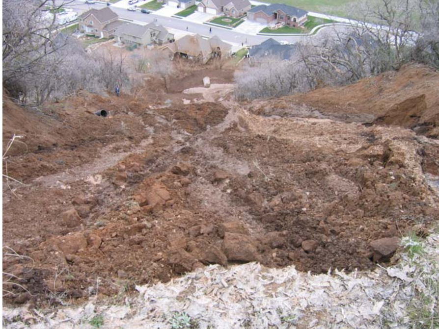
Figure 7. View looking down the landslide flow path at the damaged house at 1650 East 7687 South. The culvert in the lower slide path above the house was originally in the gravel pit. Subsequent water flow eroded the right side of the landslide.
