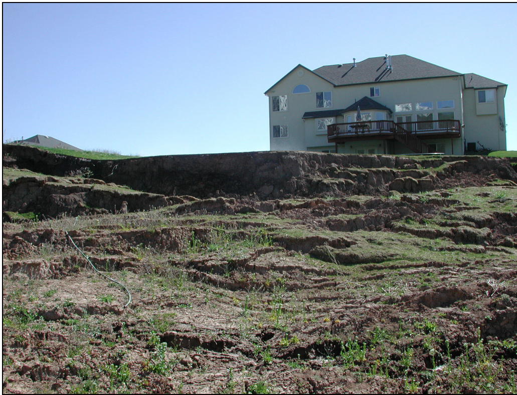
Figure 4. Damage to the rear of a lot caused by movement of the Frontier Drive landslide, Mountain Green in 2001. Losses and stabilization costs of this landslide exceeded $750,000.
