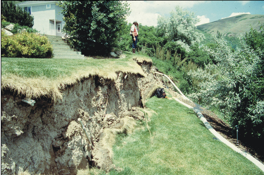
Figure 1. Damage caused by movement of Capitol Boulevard-City Creek landslide to rear of lot at 1000 E. Capitol Boulevard, Salt Lake City in 1998.
