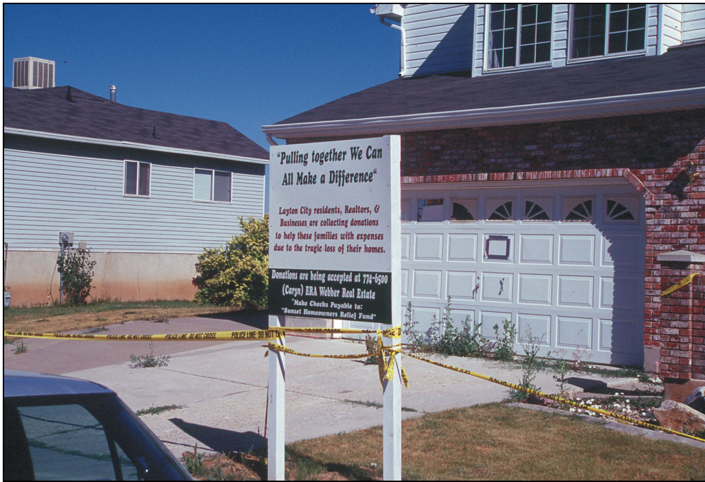
Figure 6. Two houses damaged by movement of the Sunset Drive landslide, Layton in 1998. House on the right was subsequently condemned and demolished.
