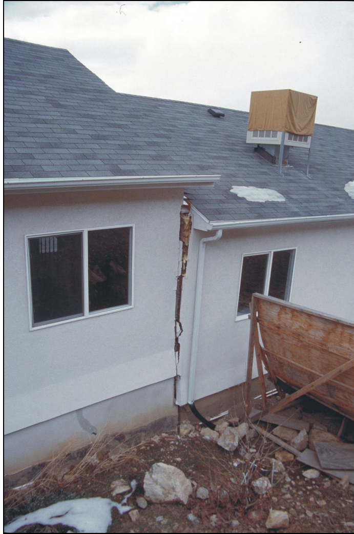
Figure 3. Damage to a house caused by movement of upper part of the Sherwood Hills landslide in Provo. House was condemned in January 2000.
