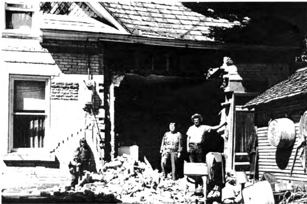
Damage to an unreinforced brick house in Richmond in the 1962 Richmond earthquake (photo by Ariel D. Benson, Richmond, Utah).
