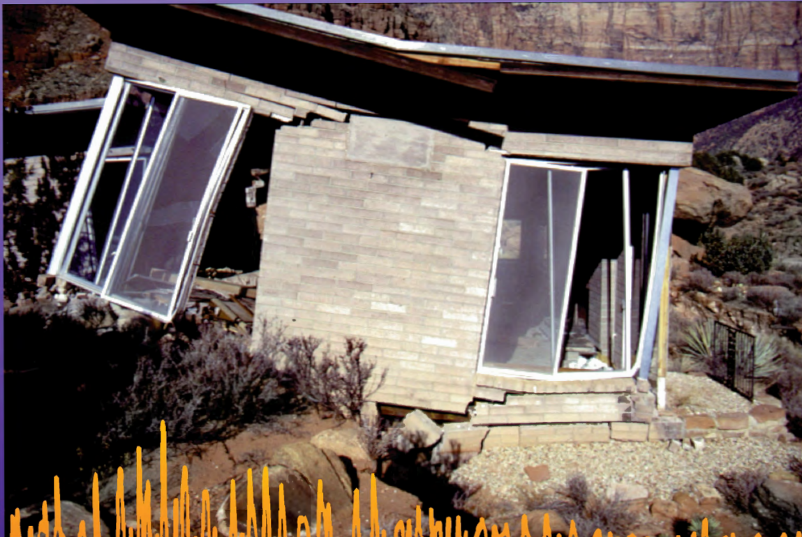
Home damaged by the landslide generated in Springdale, Utah during the 1992 St. George earthquake.
