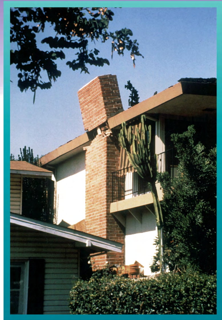
Ground shaking commonly causes chimney damage (Earthquake Engineering Research Institute).
