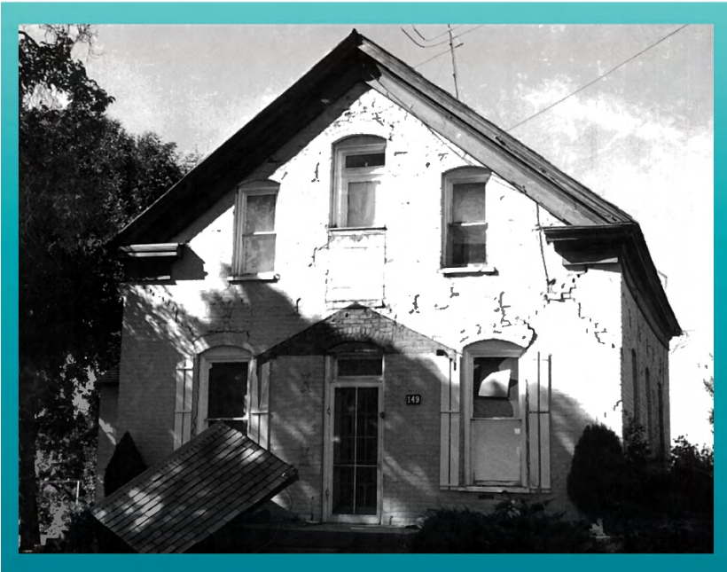
Cracking and porch-roof damage to a home in Richmond, Utah caused by a magnitude 5.7 earthquake in 1962 (Ariel D. Benson).
