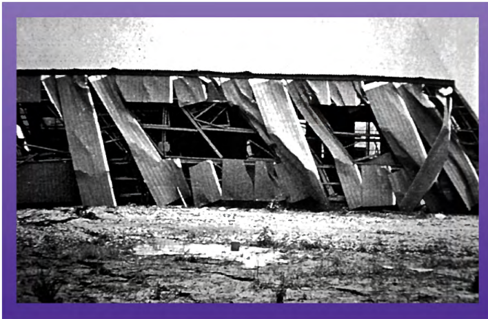
Lateral spreading tore this building apart in the 1971, magnitude 6.7 San Fernando, California earthquake (T. Leslie Youd).
