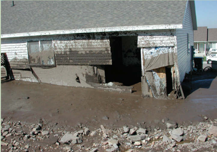
Impact from the 2002 Santaquin debris flow broke the back wall of this house, filling it with debris.
