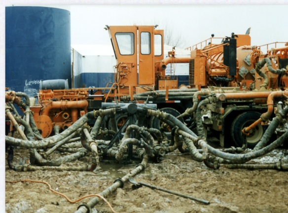
Recompleting the Michelle Ute 7-1 well. Connections from the multiple pump trucks prepared to pump acid down the well.
