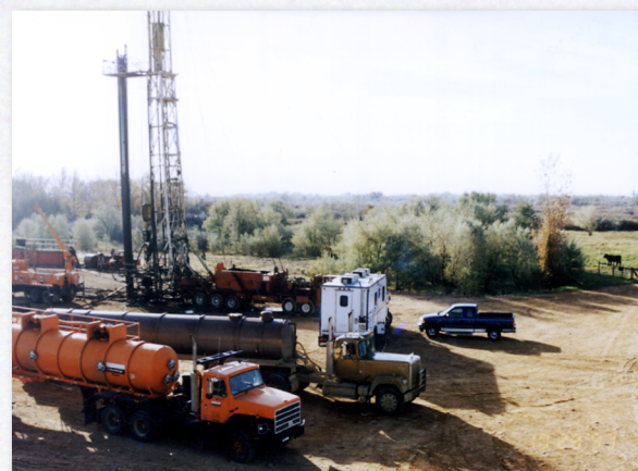
Recompleting the Malnar Pike 17-1 well. Small rig is used to pull the production tubing from the well, then the pump trucks are connected to the wellhead. The white truck is the control unit shown in upper left photo.
