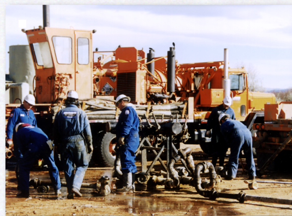
Recompleting the Malnar Pike 17-1 well. Connecting the lines that go from the pump trucks to the wellhead.
