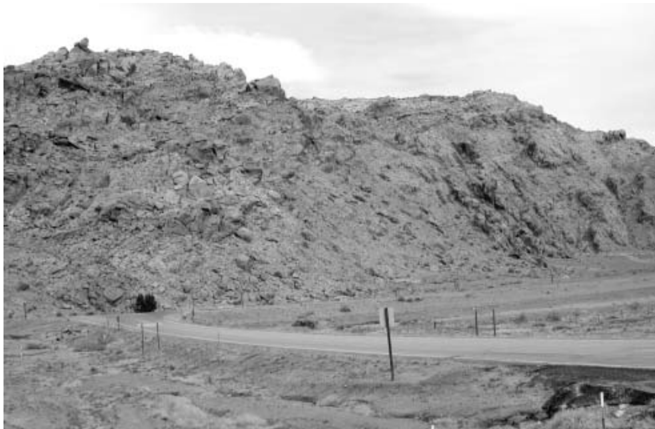
Figure 10. Highly fractured Navajo Sandstone exposed at the northwestern end of Moab-Spanish Valley, at the intersection of Utah Hwy. 279 (foreground) and U.S. Hwy. 191 (at base of slope). Fractured rock such as this poses a variety of problems for development.
