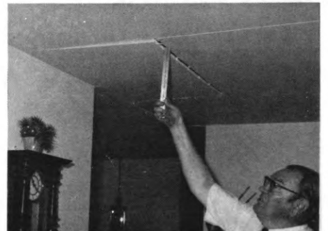
Raymond L. Hansen, Utah Dept. of Contractors representative in Ogden, measures distress evident in home interior.
