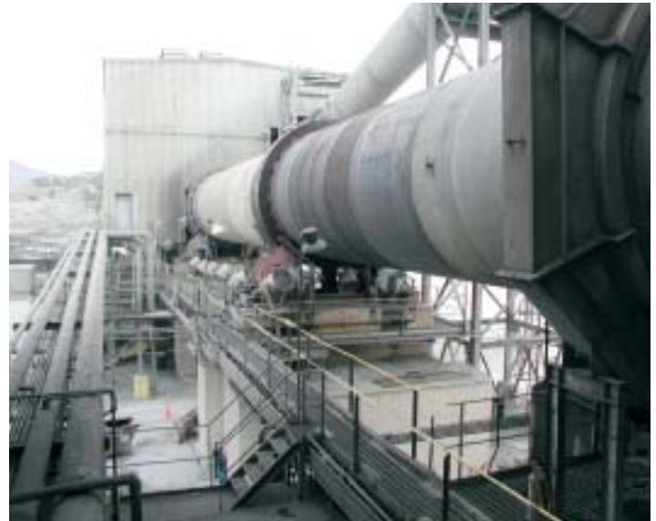
View along Leamington’s 175-foot-long, 12.5-foot-diameter rotary kiln where powdered coal is burned at about 2,650 degrees Fahrenheit to finish the chemical reactions necessary to create Portland cement.
