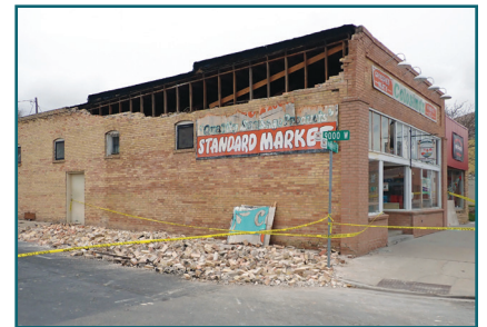
Structural damage to a building in downtown Magna caused by the 2020 M5.7 earthquake.
